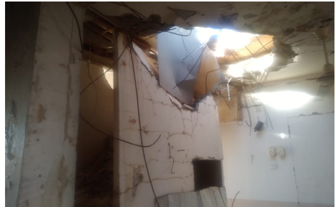
Figure 4: Damage to roof of one of the houses in Akashat
