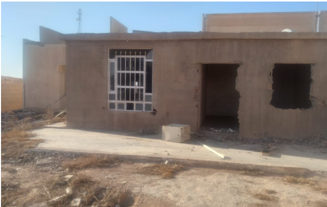
Figure 5: Picture of damage to housing shared by FGD participant
